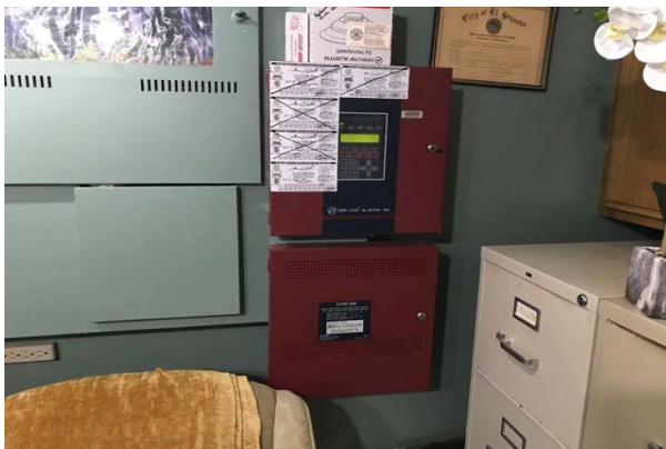
#29 FIRE ALARM CONTROL PANEL
