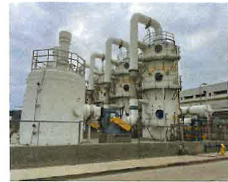
Intermediate Pumping Station BTf
