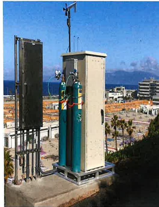
FENCE LINE MONITORING EQUIPMENT
