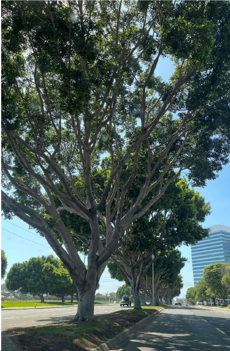
Before: Ficus trees uprooting pavement
